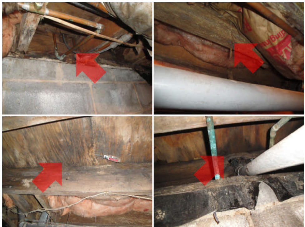
Noted significant damage to floor structure in multiple areas in crawlspace above the back, left, and front foundation walls, as well as, throughout the crawlspace. Crawlspace should be further evaluated thoroughly and repaired as needed by a licensed general contractor.
