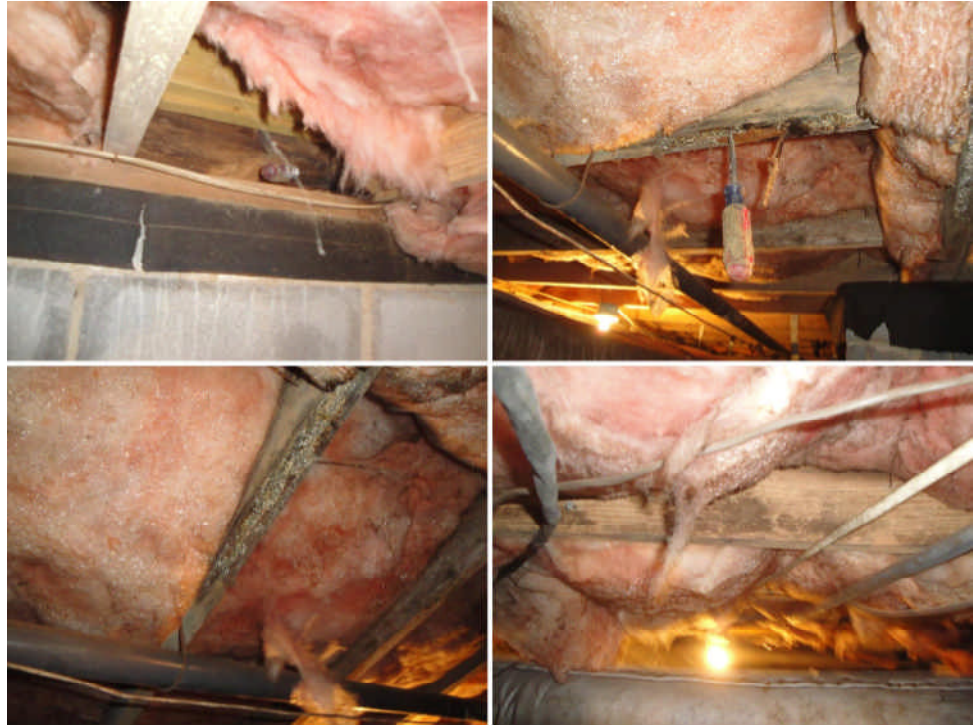
There are no readily visible problems noted in foundation. Pictures above and below show concerns in first floor structure.
